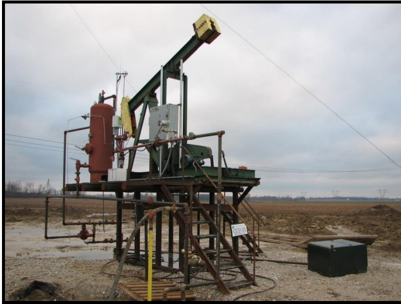
Figure 8 - Beam Pump Installed on Flood Plain in New Albany Shale Region, Illinois Basin 4
