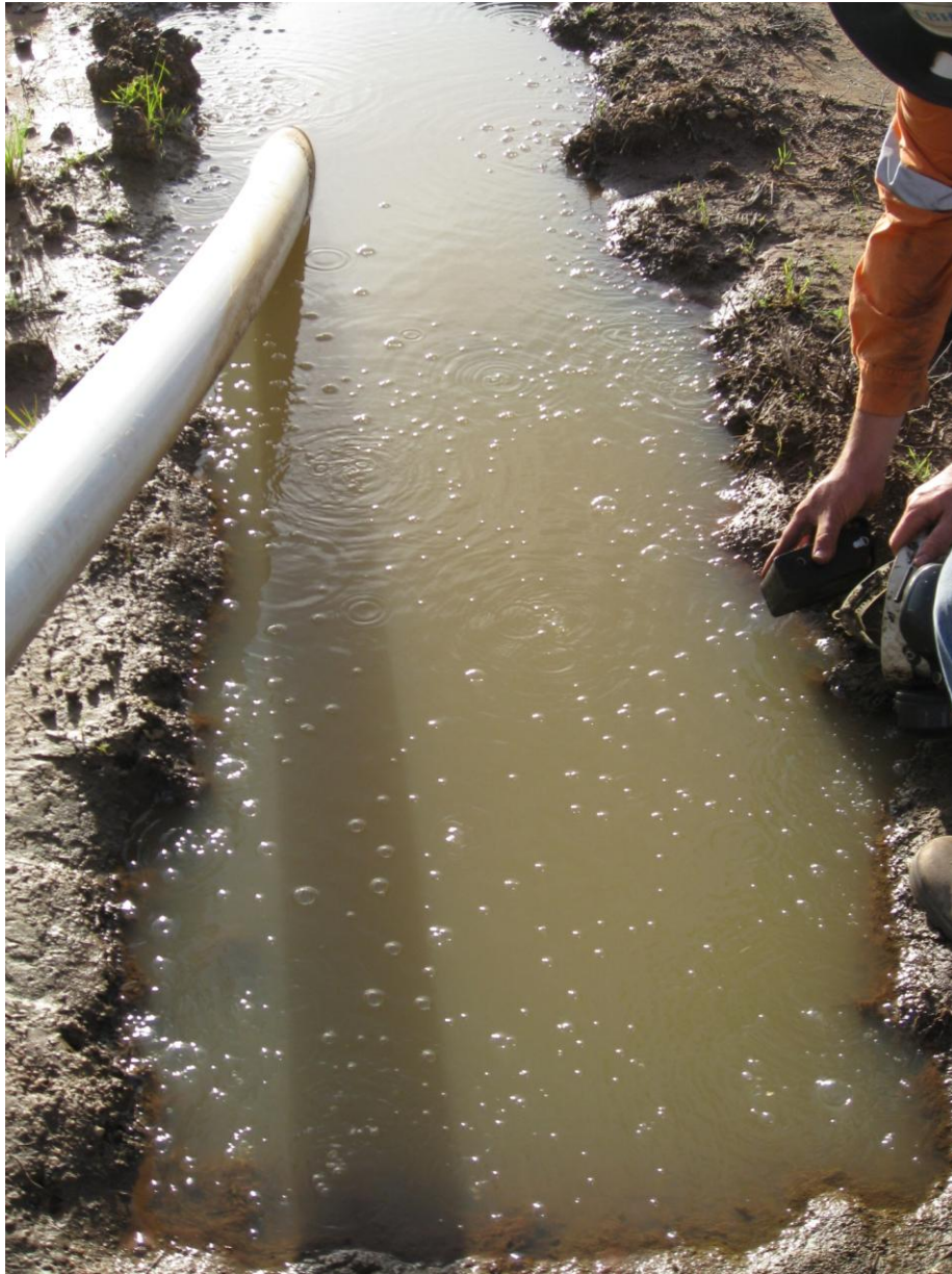
Figure 9. Gas bubbles evident in the nitrogen pipeline trench at VPW29.
