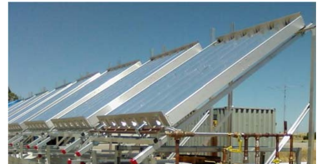
High-Temperature Solar Thermal for Steam Generation, Process Heat and Cooling
