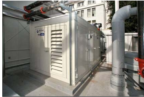
Waste Heat Chiller/Heater
