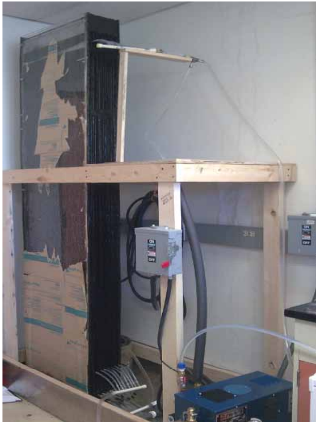
Direct steam injection
