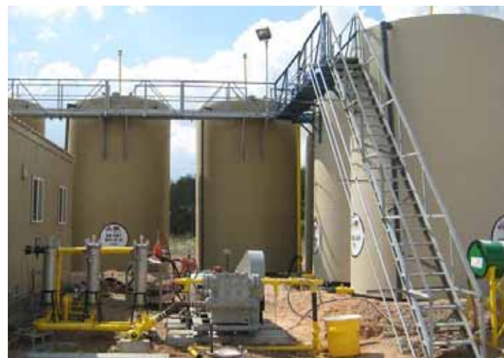
Chemical storage, mixing, filtering & pumping
