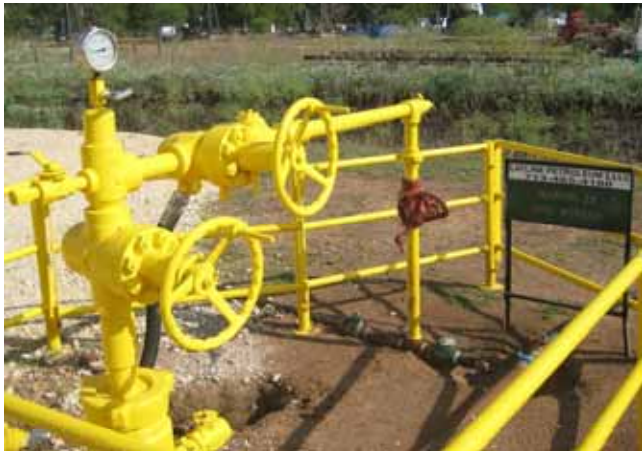
Injector (M24) wellhead
