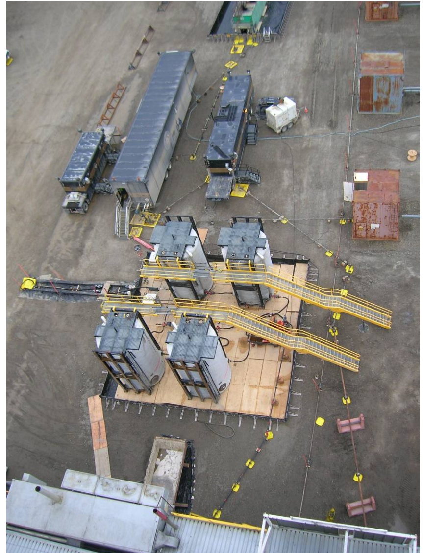
Diesel Tanks, Heater, Separator
