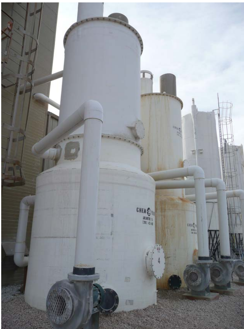
Ion Exchange Produced Water Treatment System (Montana)
